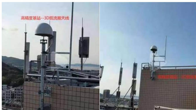
The largest 5G+ Beidou CORS station in China -- China Mobile Project
